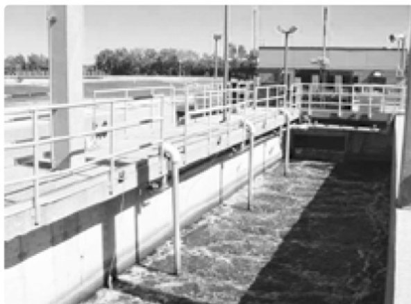
The amount of dissolved oxygen in an aeration tank is controlled by mechanical or diffused aeration. Photo courtesy of Lorene Lindsey.
