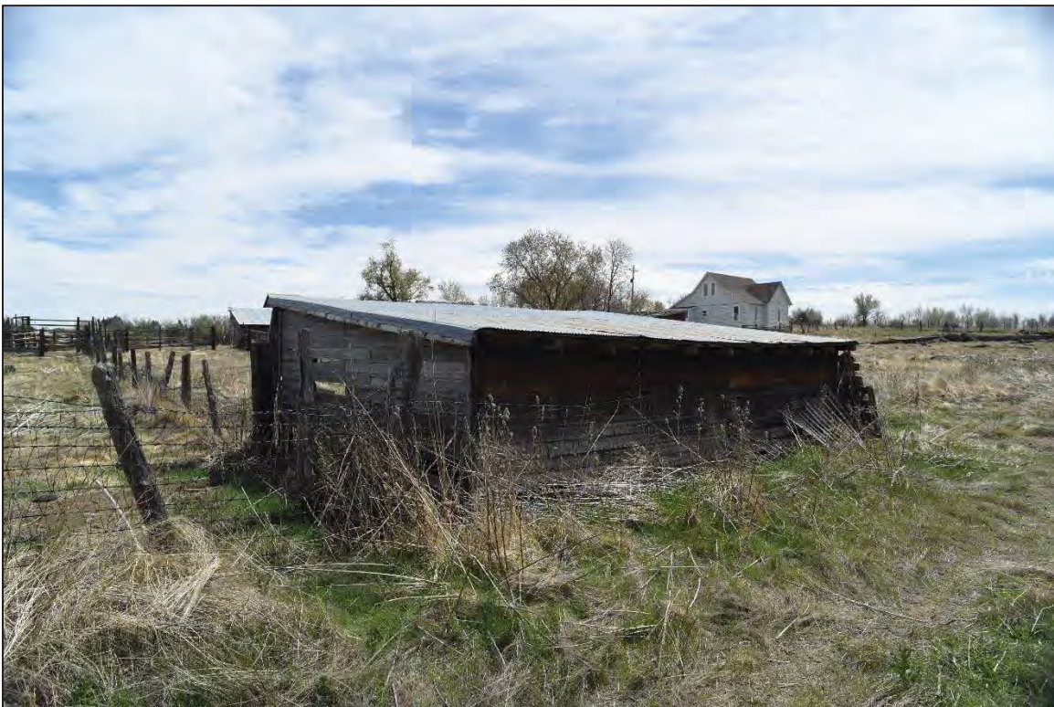
Photo 6187: Oblique view of the eastern and northern elevations of the Bull Shed.
