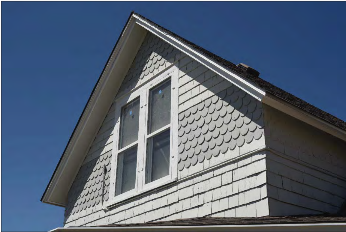
Photo 6240: Second story of the southern elevation showing decorative siding shingles on Farm House.
