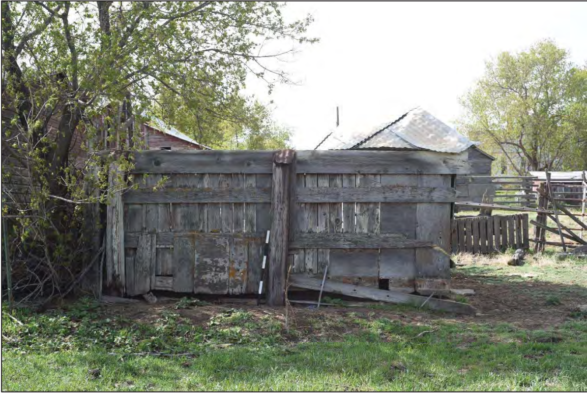
Photo 6396: Northern elevation of collapsed section of Loafing Shed .
