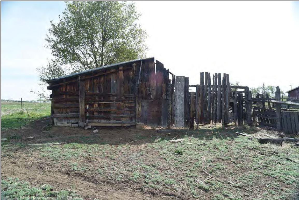
Photo 6398: Western elevation of Loafing Shed , featuring collapsed section.
