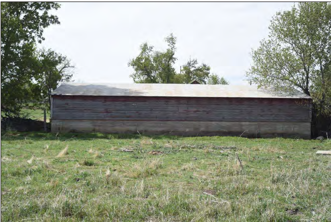
Photo 6392: Northern elevation of Loafing Shed . The collapsed section of the loafing shed is not visible and is separate from the main section by the tree visible on the right edge of the frame.
