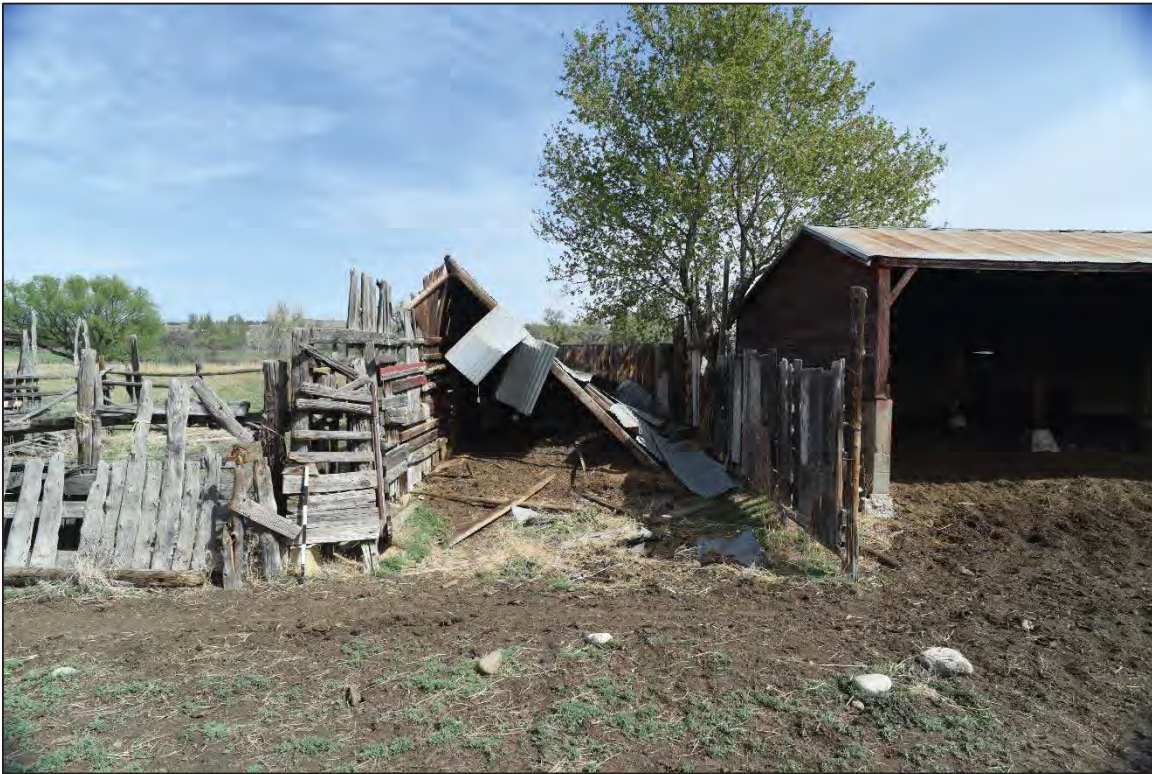
Photo 6403: Overview of collapsed Loafing Shed section from the south.
