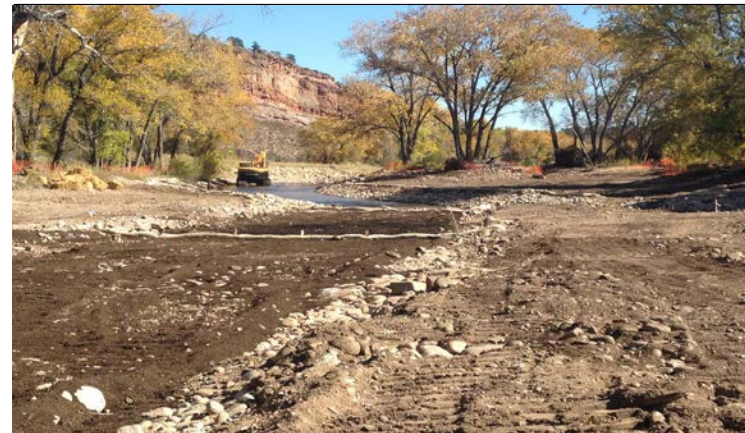
Downstream View: Buried rock ramp and confluence of overflow channel A and main channel.
