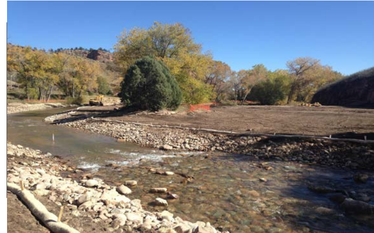
Downstream View, Right bank: Creek platform, floodplain benching, fine grading and soil conditioning between main St. 84+50 to 88+00.
