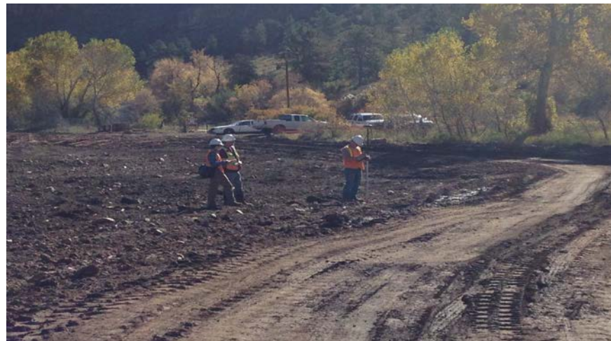
Spot checks and grade verifications of right flood plain between St. 74+00 to 82+50.
