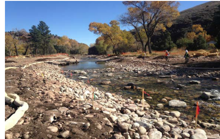
Downstream View: Boulder toe bank stabilization with cobble as filler and face material between main channel St. 92+94 to 94+30 left bank.
