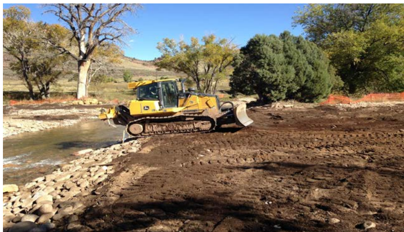
Downstream View: Soil Conditioning in progress in right floodplain adjacent to main channel St. 86+50.
