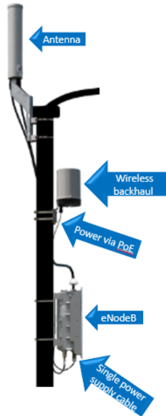
Figure 17 An example of small cell pole deployment with only power supply is required to the pole
