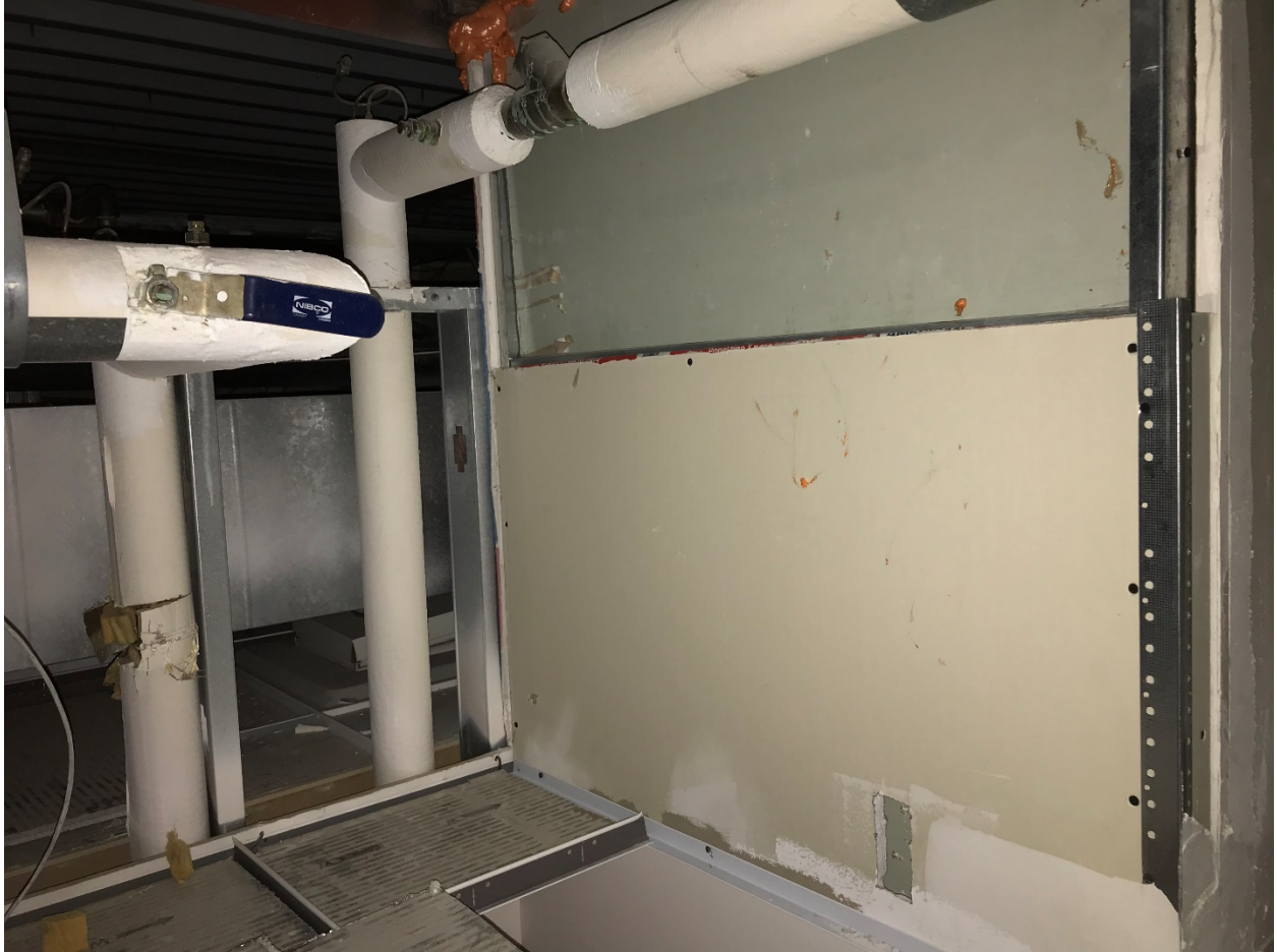
Hot Water Pipe at 3 rd floor ceiling See Note 9 on M1.1
