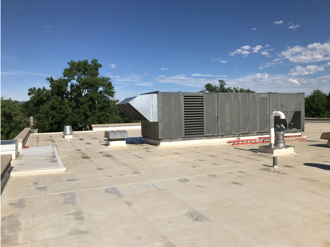
East Side AHU
