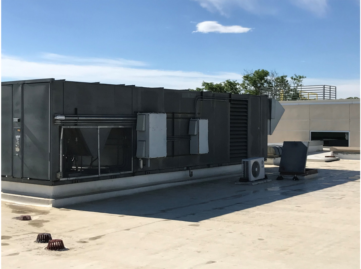
West Side AHU
