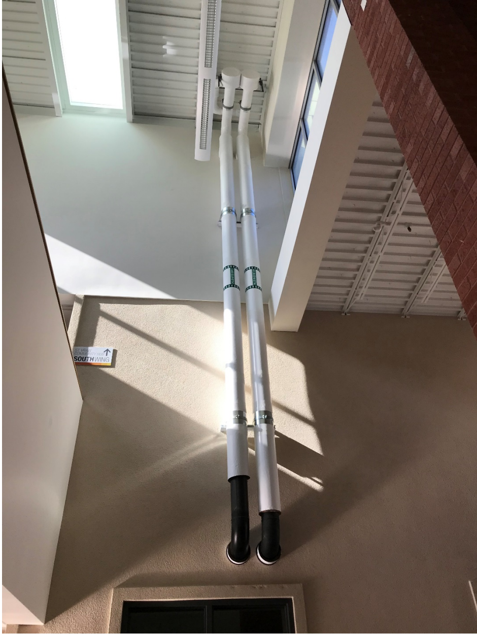
Atrium Chilled Water pipe. See Note 4 on M1.1
