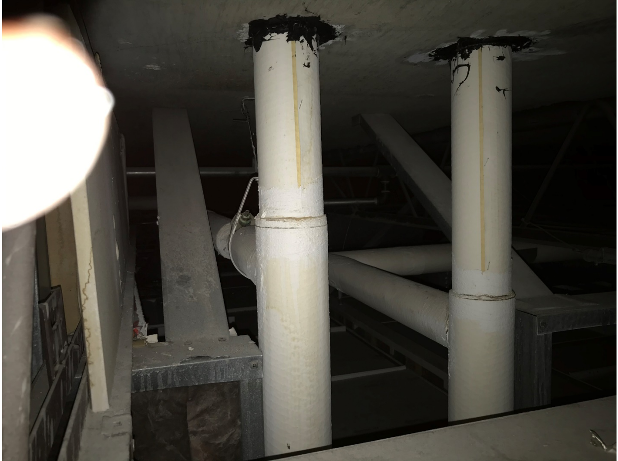
Hot water pipe at 2 nd floor ceiling. See Note 9 on M1.1
