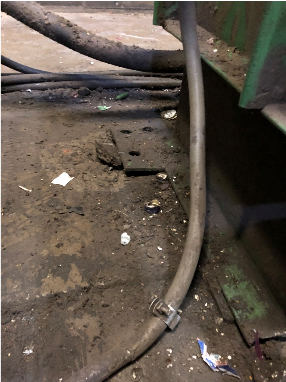
Bolts missing from floor plate
