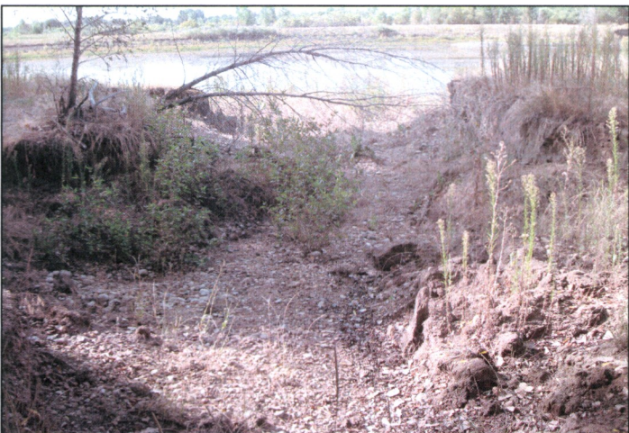
5. Bank erosion of eastern pond.
