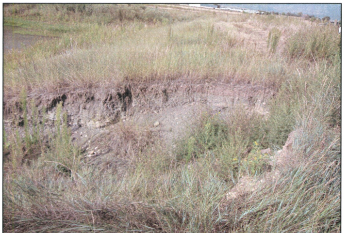
6. Bank erosion of eastern pond.
