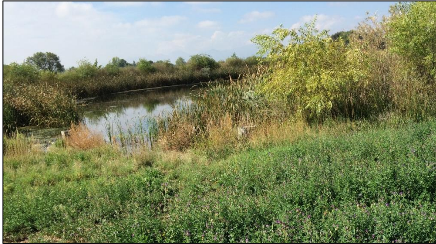
Photo 40. View of pond 9 from northern shoreline in area south of river. Pond slopes are at 3H:1V or flatter with good vegetative cover.
