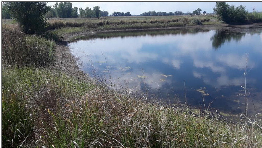
Photo 26. View of eastern shoreline of pond 4 in area south of river. Pond slopes are at 3H:1V or flatter with good vegetative cover.
