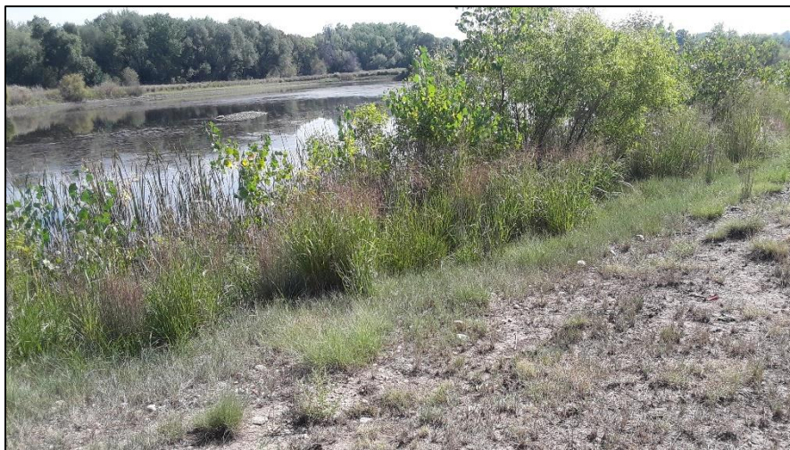
Photo 24. View of southwestern shoreline of pond 4 in area south of river. Pond slopes are at 3H:1V or flatter with good vegetative cover.
