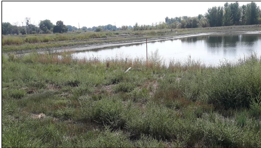
Photo 29. View of eastern shoreline of pond 5 in area south of river. Pond slopes are at 3H:1V or flatter with good vegetative cover. Kochia covers much of grasses along northern shoreline (foreground).
