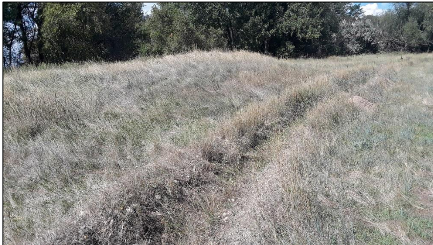
Photo 14. View of berm separating ponds in north area from river, which appeared to be stable with good grass cover.
