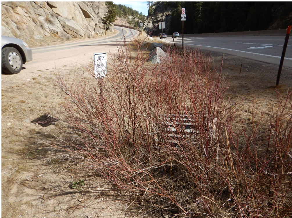
Photo 6. Looking east at a storm drain at the west end of the study area.
