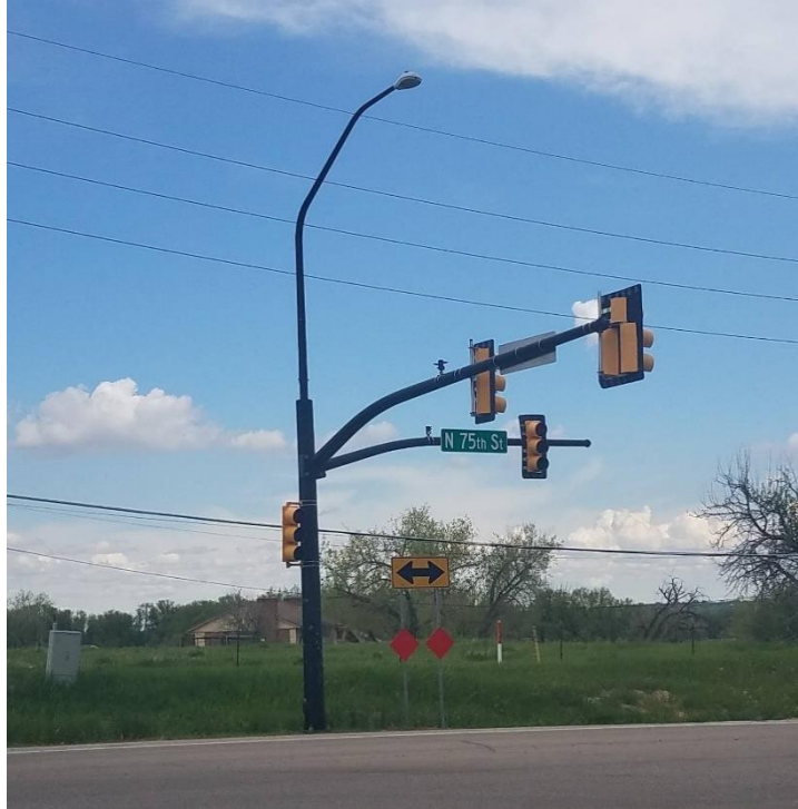
Signal Pole w/ Two Mast Arms and Luminaire Arm (N 75th Street and Jay Road)
