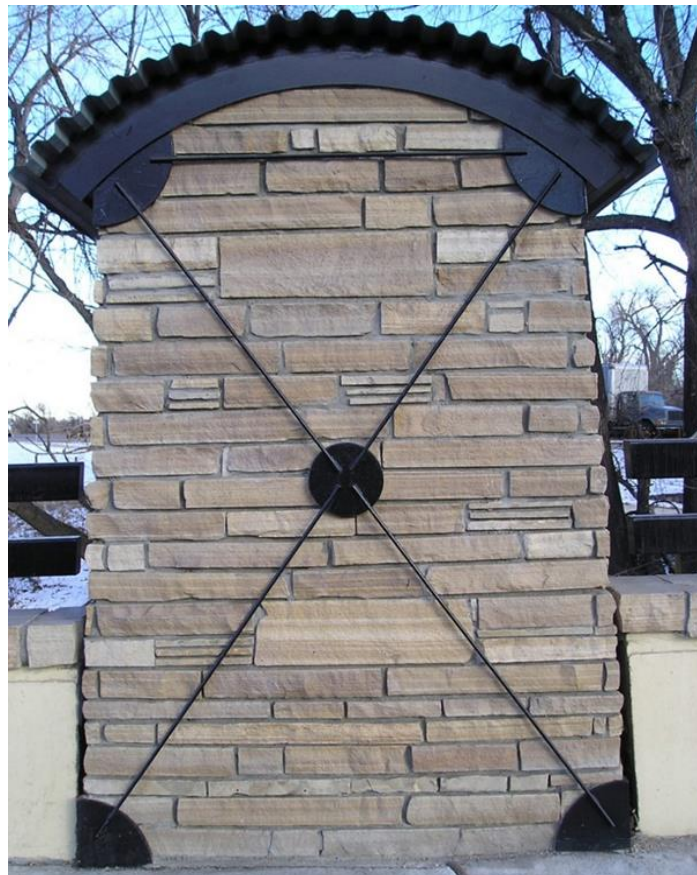
Photo (circa 2004) showing ironworks (facia plates, cross-rods) on pilaster, painted semi-gloss black
