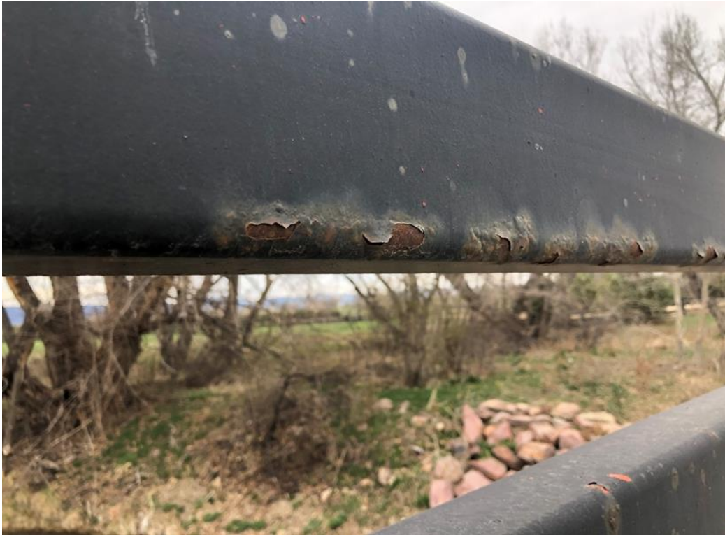
Corrosion on bicycle rails (current photo)
