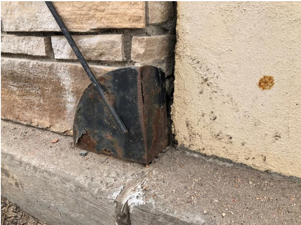
Current photo showing flaking, chipping, corrosion of ironworks fascia on pilaster
