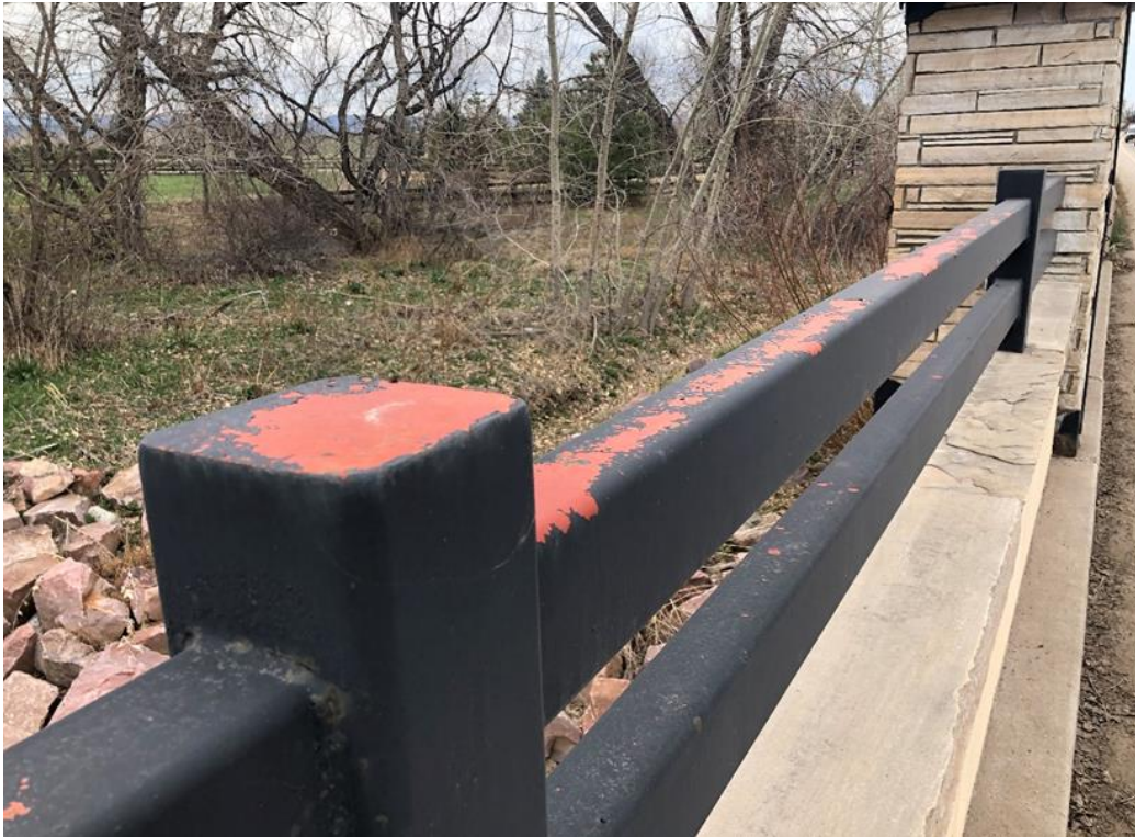
Example of chipped, flaking paint on bicycle rails (current photo)
