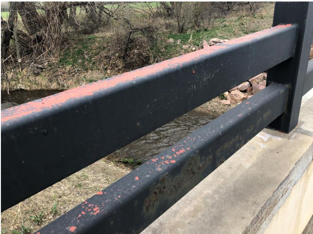
Chipped, flaking paint and corrosion (current photo)
