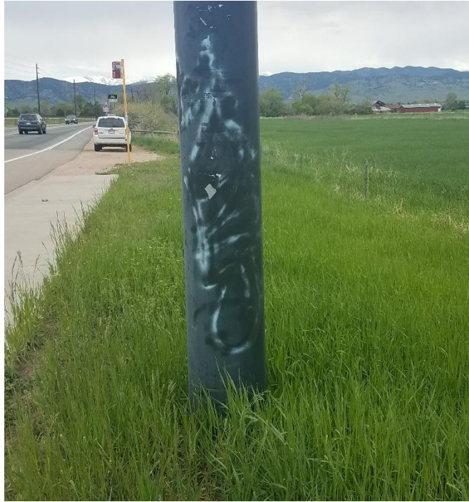
Paint Fading with Graffiti
