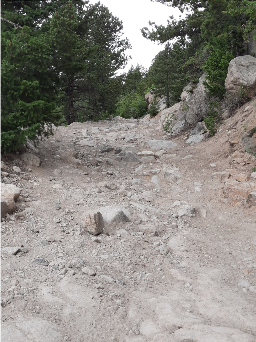
Access road above first switchback above Peaceful Valley Campground.
