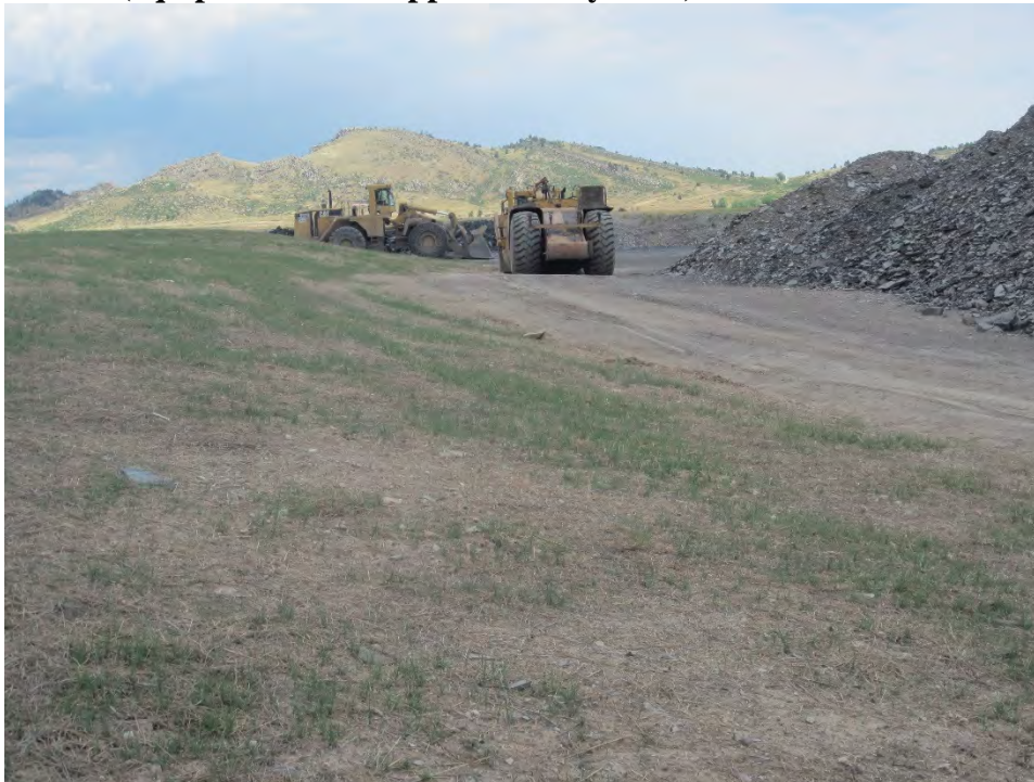
Figure 1: 2014 reclamation with over 6-ft of compacted subsoil for potential prairie dog habitat (equipment tire is approximately 12-ft)
