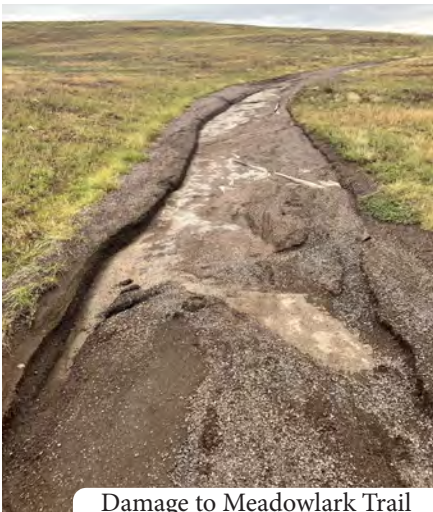
Damage to Meadowlark Trail
