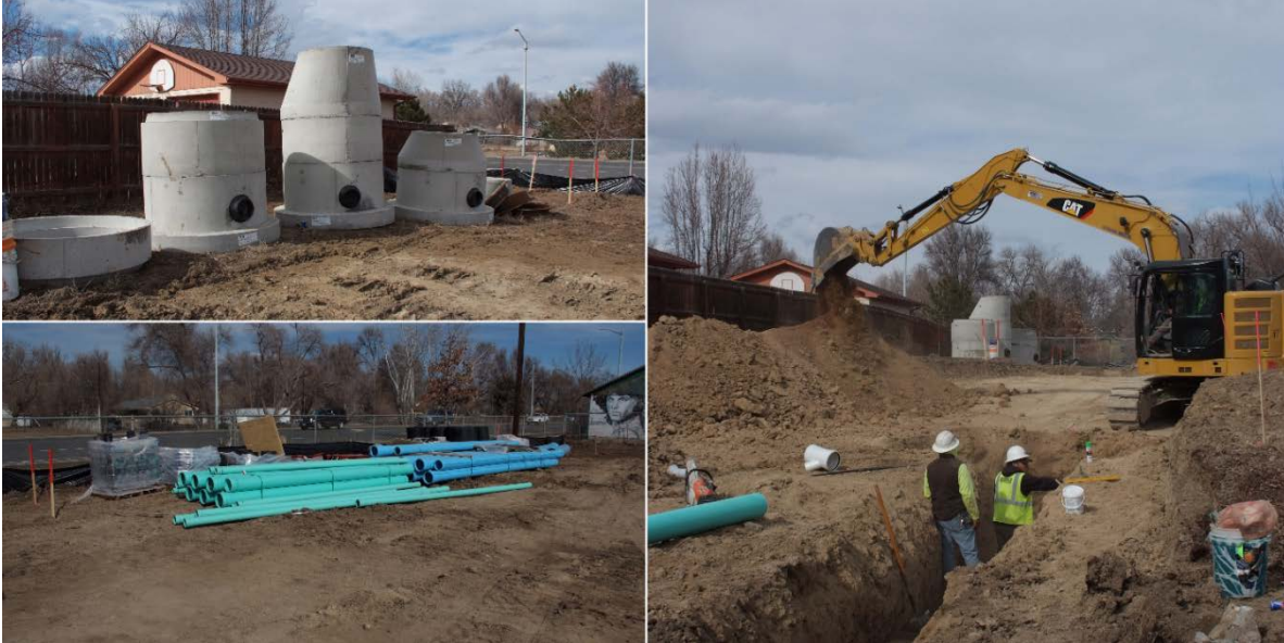
East Rogers Road Development project being built by Habitat for Humanity of St. Vrain Valley
