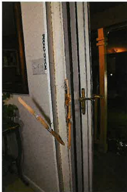
The door frame had damage to it caused by the officers' entry.
