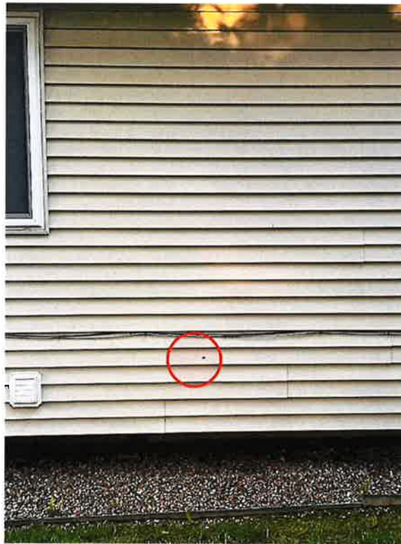
Bullet hole in exterior wall of residence behind 2184 Stuart Street.
