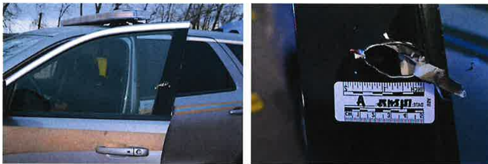
Photographs of the defect in front driver's side of the CSP vehicle
