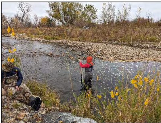
Installing a depth and temperature sensor at the Niwot Passage Project. A person in waders is standing in the river preparing to drop a depth sensor into its PVC housing, mounted on a t-post installed vertically in the stream bed. Another person in waders sits on the bank taking notes.
