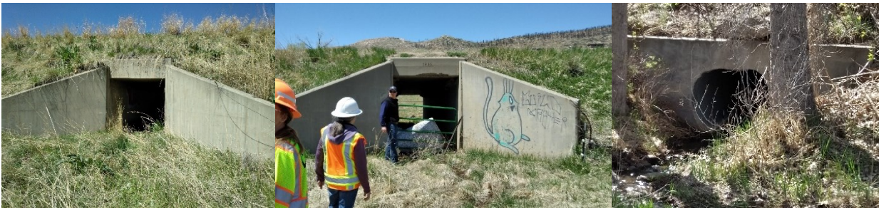
Photo 3. View of Existing Drainage Structures near MP 25.5 (Left), MP 26.8 (Middle), and MP 24.4 (Right)
