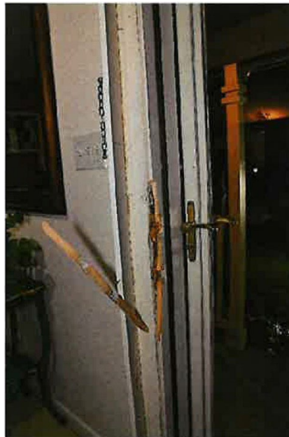
The door frame had damage to it caused by the officers' entry.
