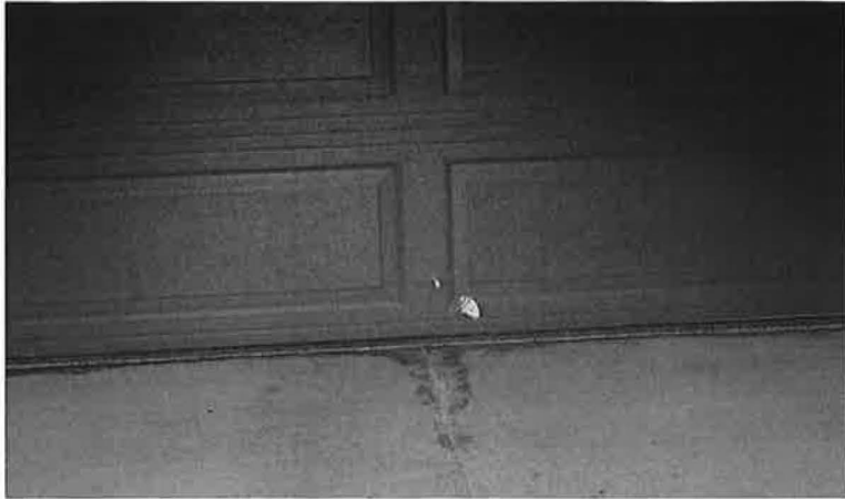
Bullet hole in exterior garage of Ms. Brownell's home
